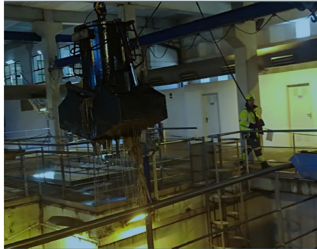
Figure 1. A metal arm removing the mass made up of accumulated cleansing wipes from Ourense's municipal treatment plant
