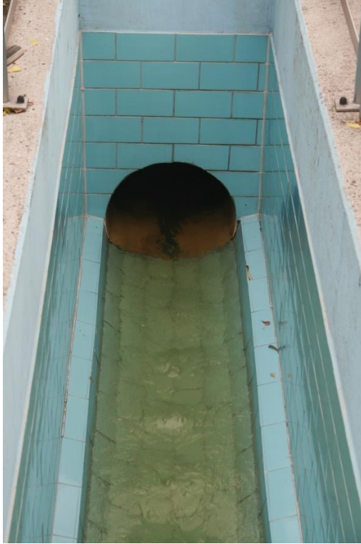
Illustration 10: Outlet pipe of the water-treatment facility
