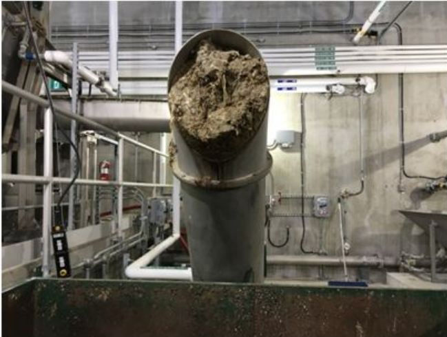
Figure 13 Image taken at Cobourg Water Pollution Control Department Treatment Plant #1, April 25, 2018: Items seen clogging the shaft, after initial screening, to go to landfill.
