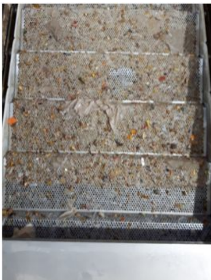
Figure 12 Image taken at Cobourg Water Pollution Control Department Treatment Plant #1, April 25, 2018: Monster™ Finescreen Separation System seen with large flushable wipes clogging the holes. In September 2017 Cobourg installed a $2 million set of new submersible pumps, to try and grind these larger items before they damage the screens.
