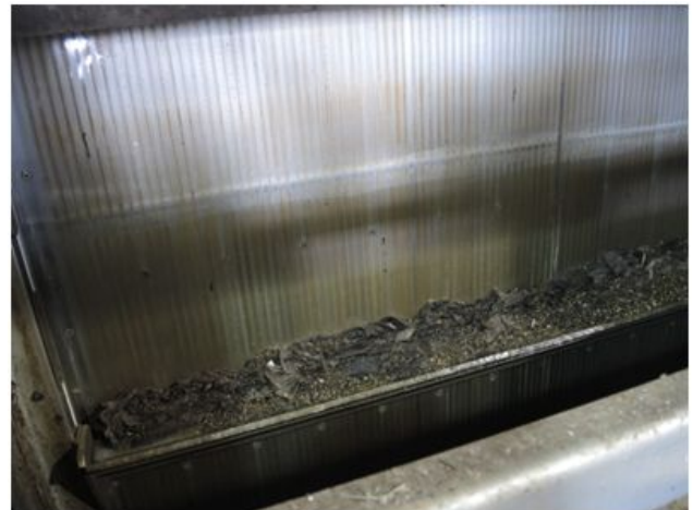
Figure 16 Image taken at Duffin Creek Water Pollution Control Plant, September 18, 2014: The initial step of the Monster™ Finescreen Separation System, bombarded with non-flushables.
