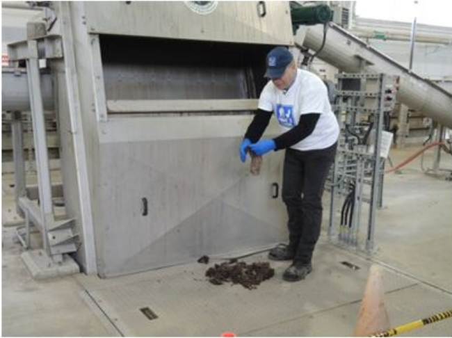
Figure 17 Image taken at Duffin Creek Water Pollution Control Plant, September 18, 2014: Barry Orr extracting non-flushables, fully intact, from the Monster™ Finescreen Separation System.
